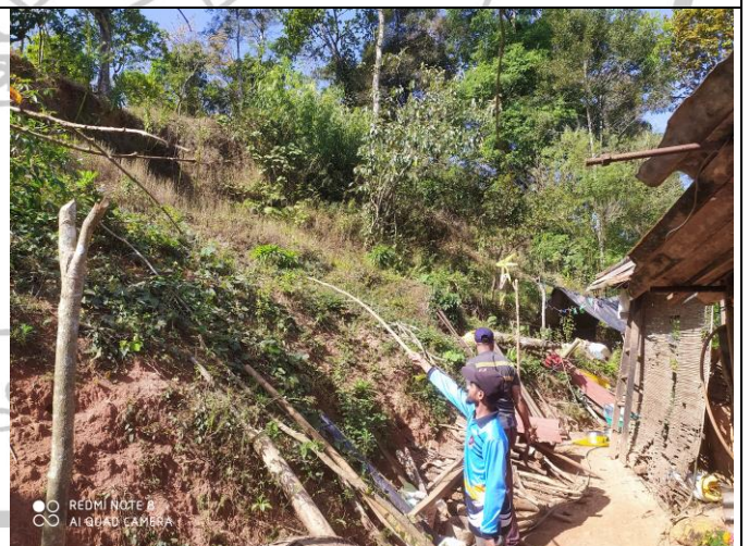
F) Cut-slope failure in Kottachi Kedhamallur village (12°09'28.16"N/75°44'9.32" E)
