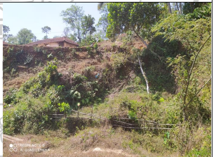
L) Debris slide occurred in Thomara village due to toe erosion (12°09'25.6"N/75°43'27.07"E)
