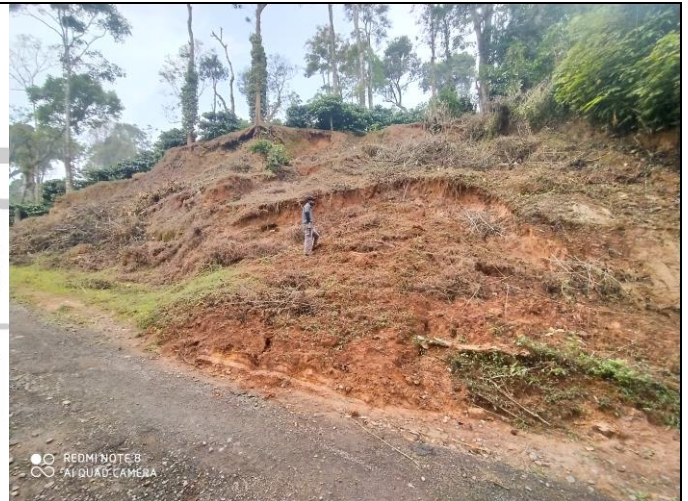
B) Cut-slope failure in Thomara village (12°10'16.89"N/75°43'27.96"E)
