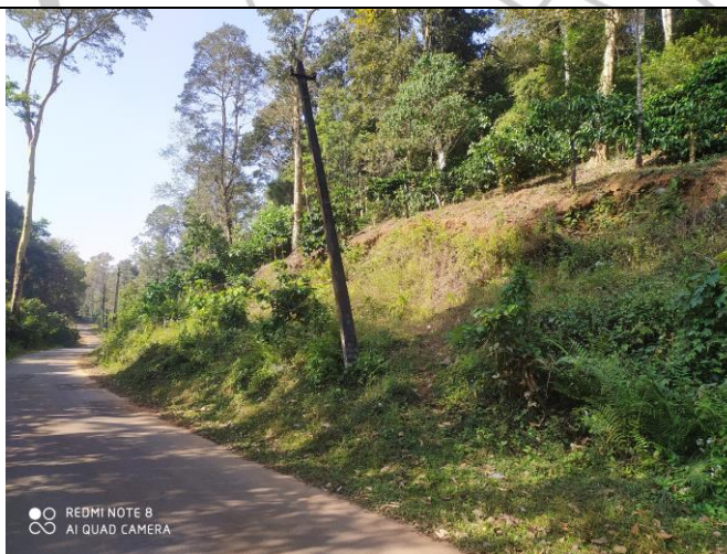
E) Cut-slope failure in Thomara village (12°09' 52.56"N/75°43' 37.27" E)
